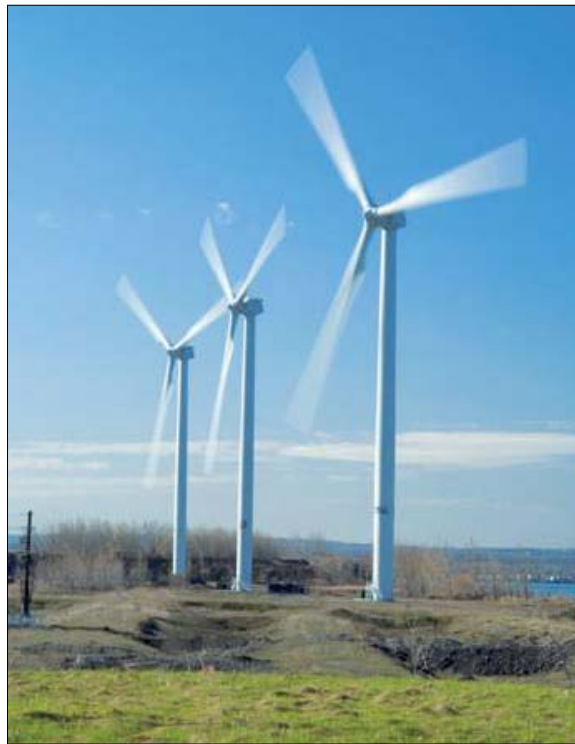
Figure 16. Liberty C96 turbines at Steel Winds (Niagara project), Lackawanna, New York
